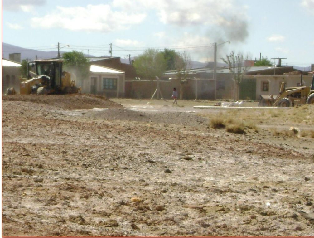
A child walks through the unprotected worksite as lead dust billows into the air due to the inadequate clean-up procedures. Abra Pampa, Barrio 12 de Octubre. José Sajama. November 18, 2011.
