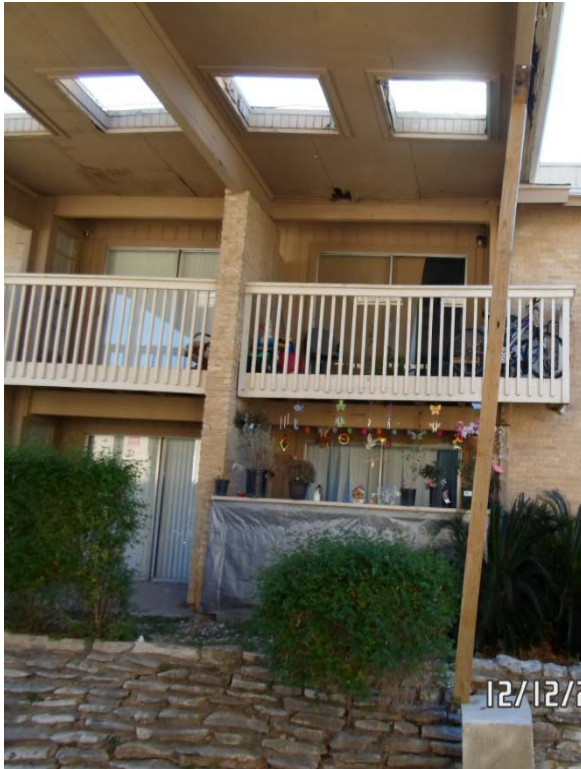
Post supporting roof is inadequate with risk of roof collapsing.
