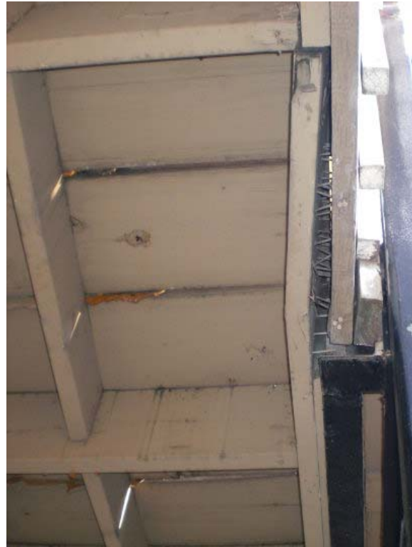
Second floor walkway becoming detached from support posts and at risk of collapsing.
