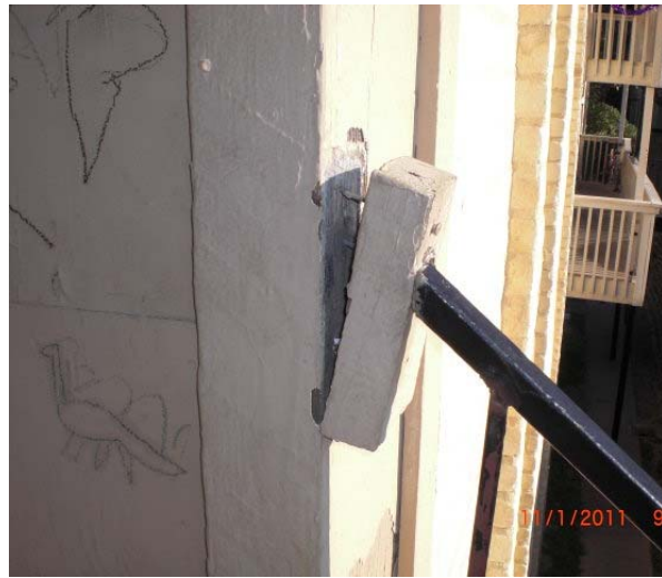
Handrail no longer anchored adequately and pulling away from structure.
