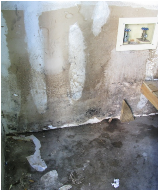
Mold on interior walls and floors.
