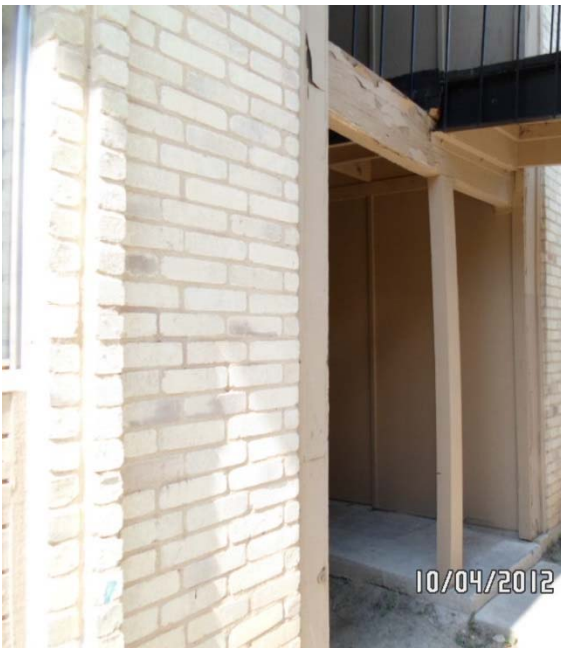
Sagging horizontal member beam and bowing support post not strong enough to carry imposed load.
